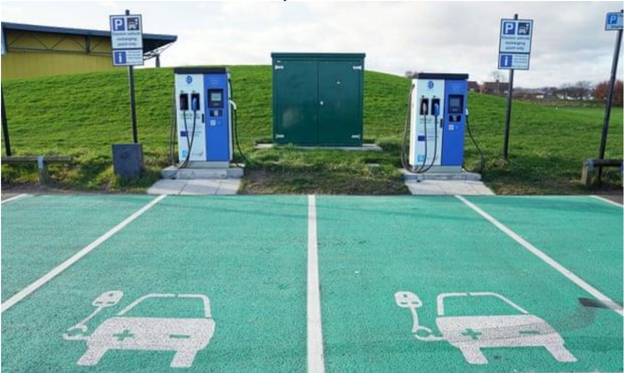
Electric vehicle charging points at Tynemouth. Photograph: Owen Humphreys/PA
